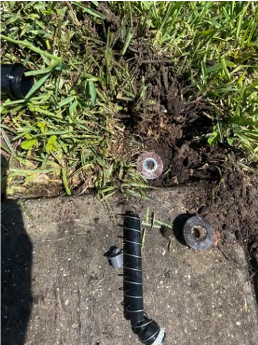
Broken pop-up on Zone B48 was replaced.
