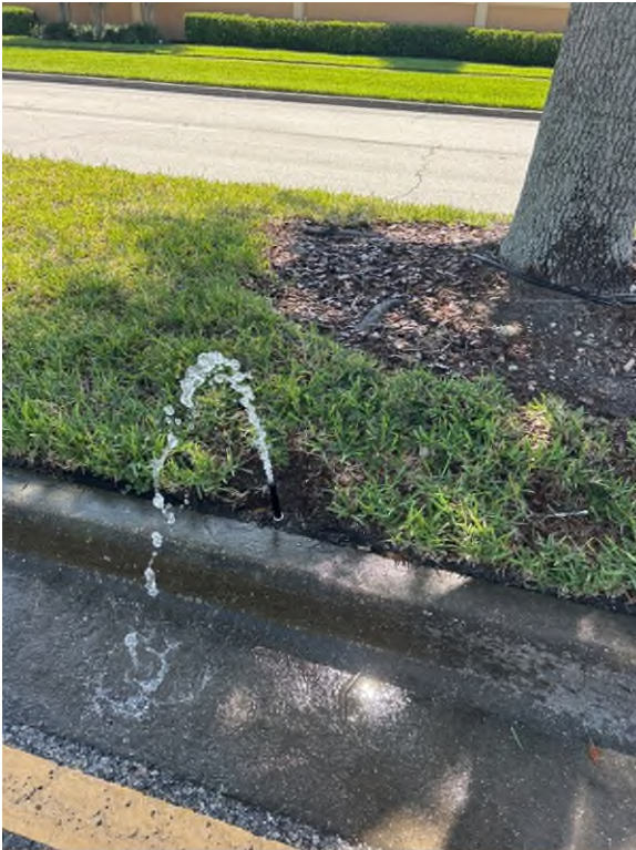
Broken pop-up on Zone B46 was replaced.
